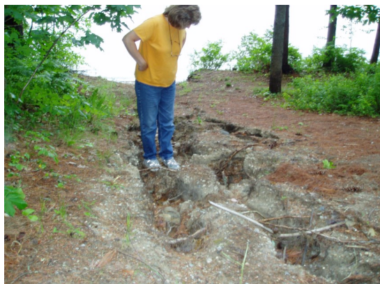
Severe erosion on a steep slope. Photo credit: Maine DEP/Portland Water District Rubber Razor Factsheet.
