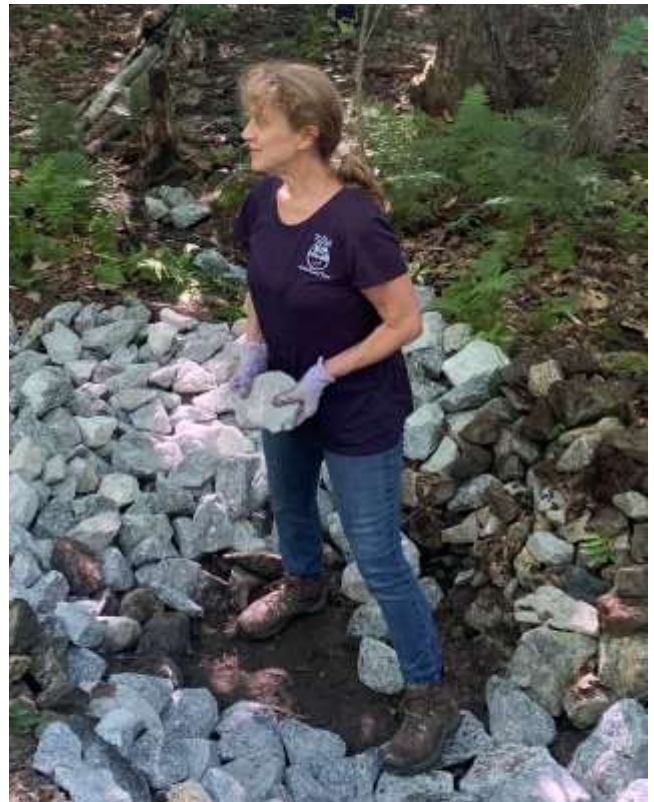
Ginger Eaton, a newly trained evaluator on Keoka Lake, assists with construction of a plunge pool to slow down runoff on a LakeSmart property.
