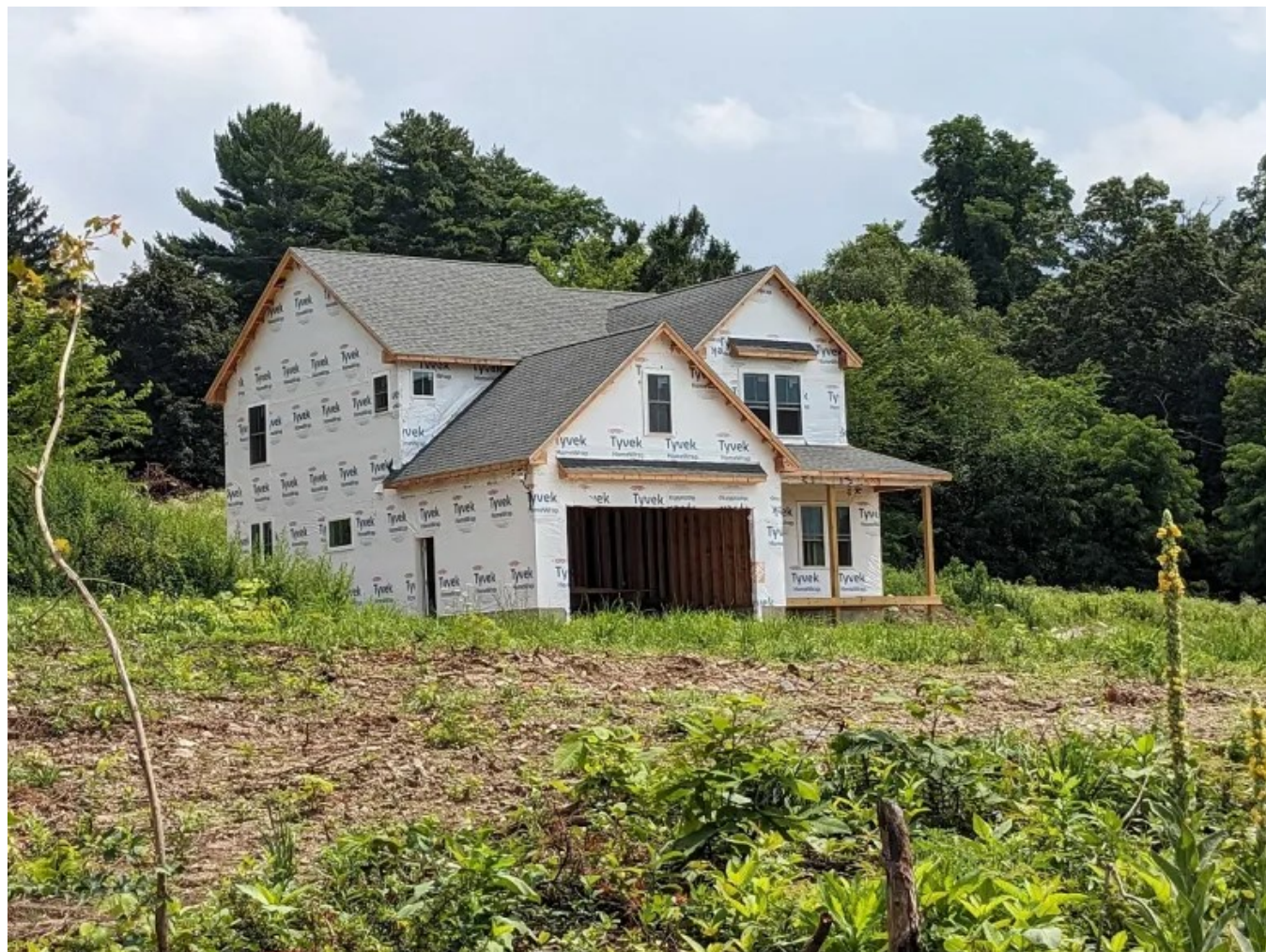
A new home under construction in Somers, Connecticut Credit: Hugh McQuaid / CTNewsJunkie
